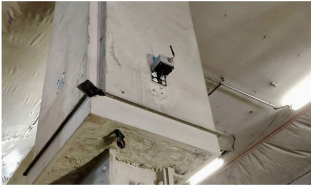
FIGURE 6 Example of tiltmeter installation for Courtesy of SIXENSE Oceania
